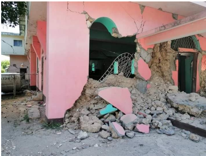
Damage to Church of Latibolière outside of Jérémie
